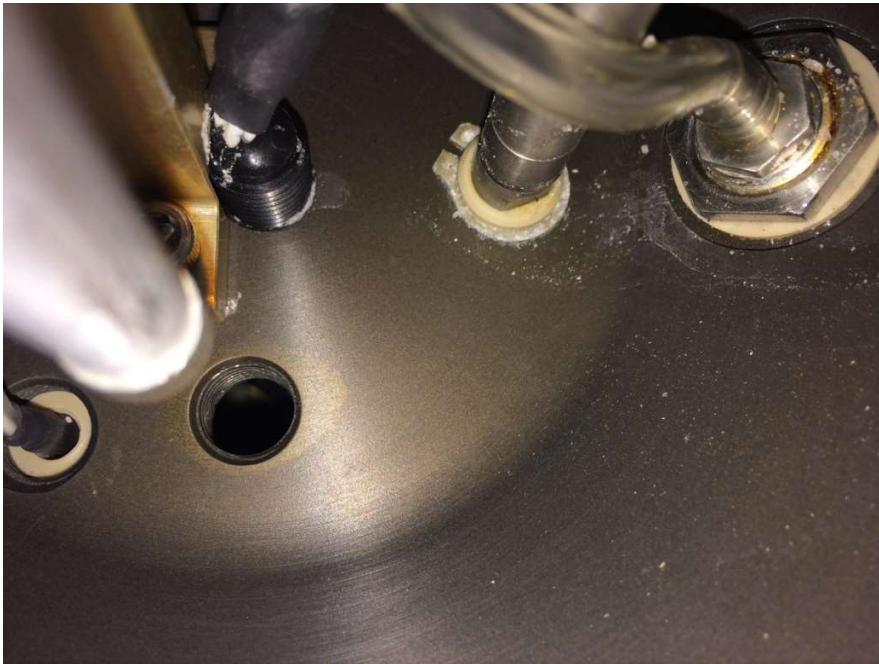
Figure 10.1.6: Trail of salt crystals in the interior of the rear bulkhead of unit 408.
