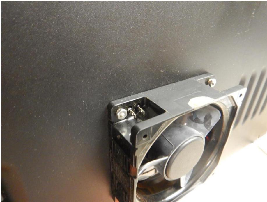
Figure 11:- Autosol S/N 65753 Disconnected Exhaust Fan
